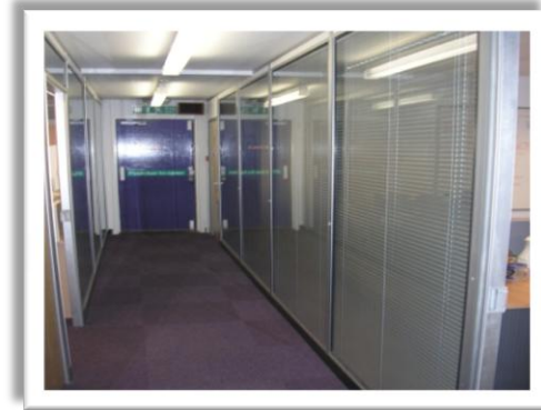
Glazed partitions with integral blinds to these offices at a Kent Power Station
